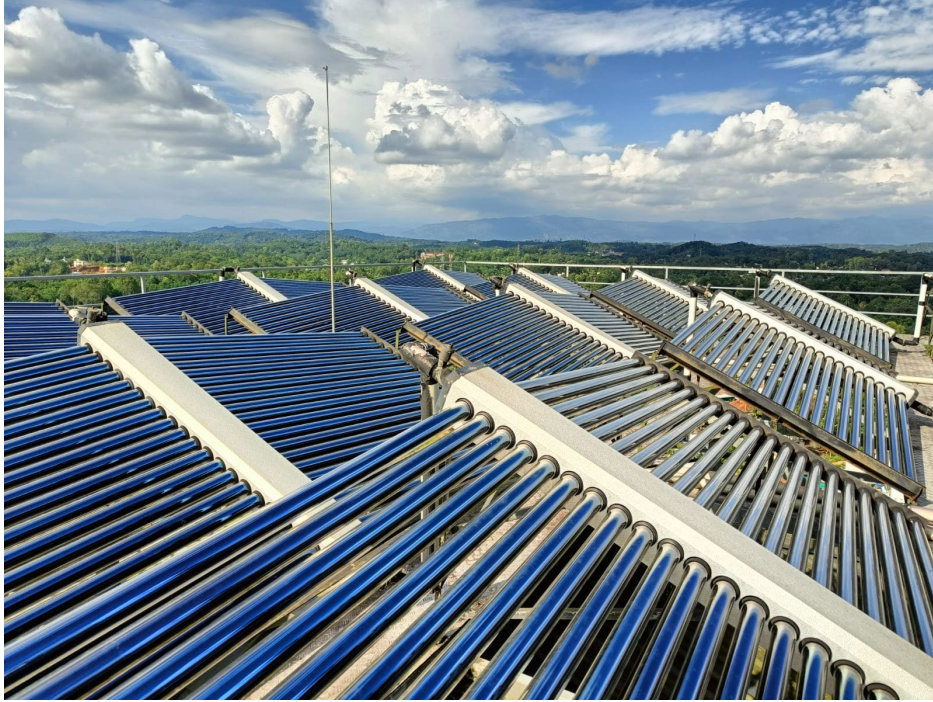
Solar water heater
